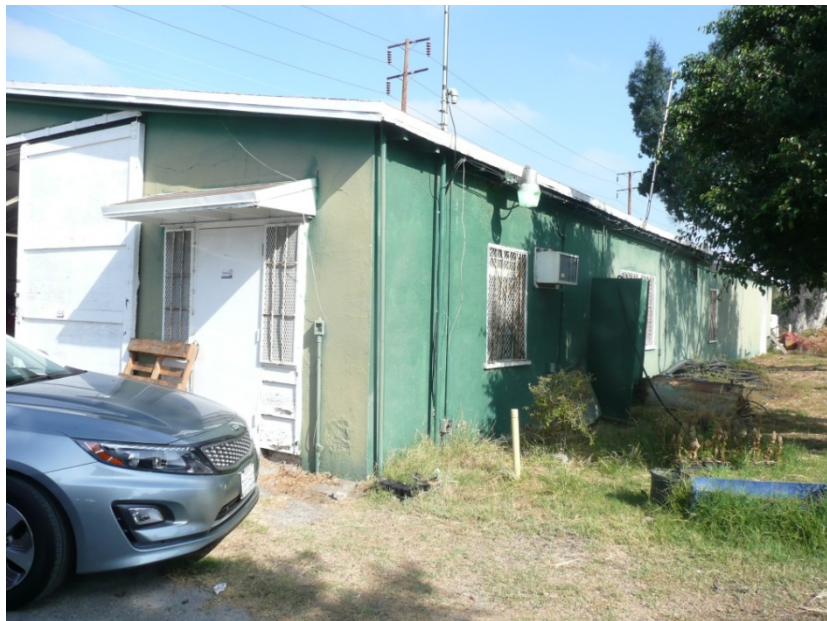
Figure 8. View of Maintenance Shed Eastern Side, Chester Washington Golf Course SOURCE: Sapphos Environmental, Inc., 2016
