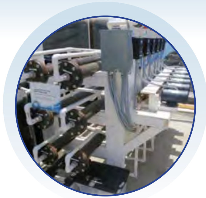
Figure 10-4: Pipe Loop Set Up
