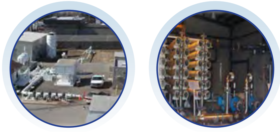
Figure 10-7: Brewer Desalter Treatment Facility
