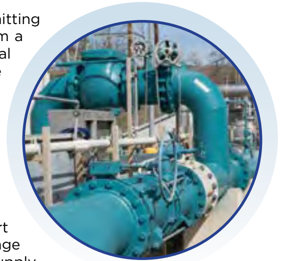
Edward C. Little Water Recycling Facility (El Segundo, CA)
