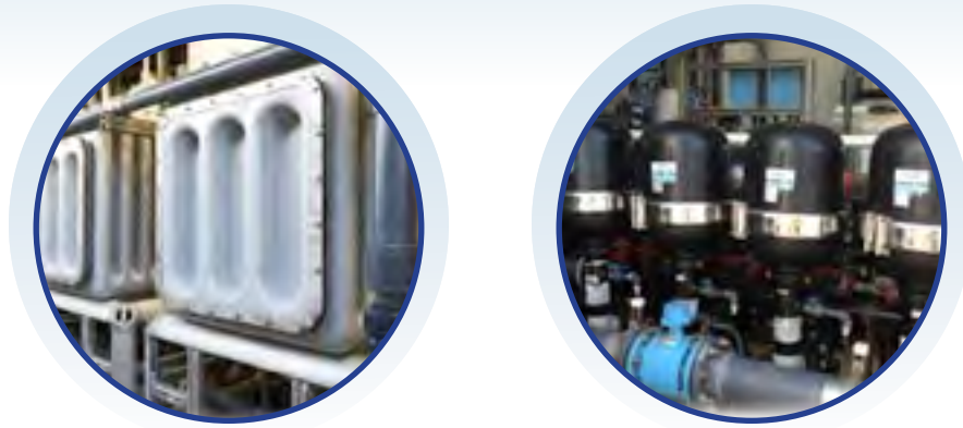
Figure 10-3: West Basin's Ocean Water Desalination Demonstration Facility
