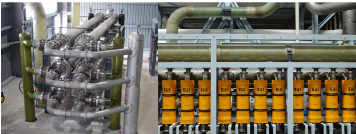
(a) Work exchangers (Calder DWEER)
