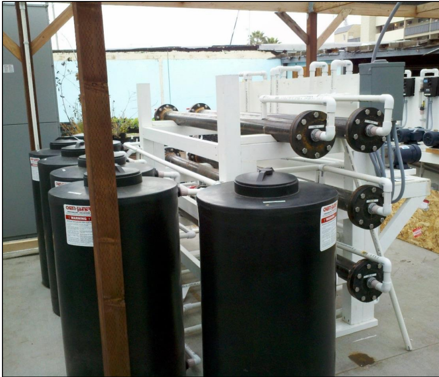
Figure 3-4. CML Pipe Loops
