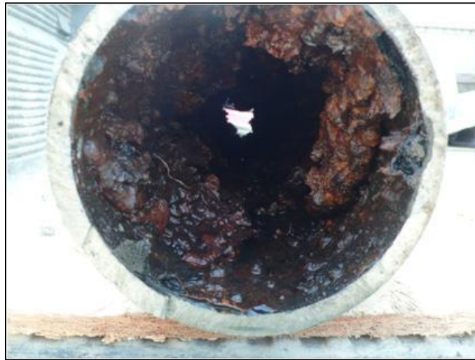
Figure 3-3. UCI Pipe Loops (top) and Cross Area (bottom) of UCI Pipe
