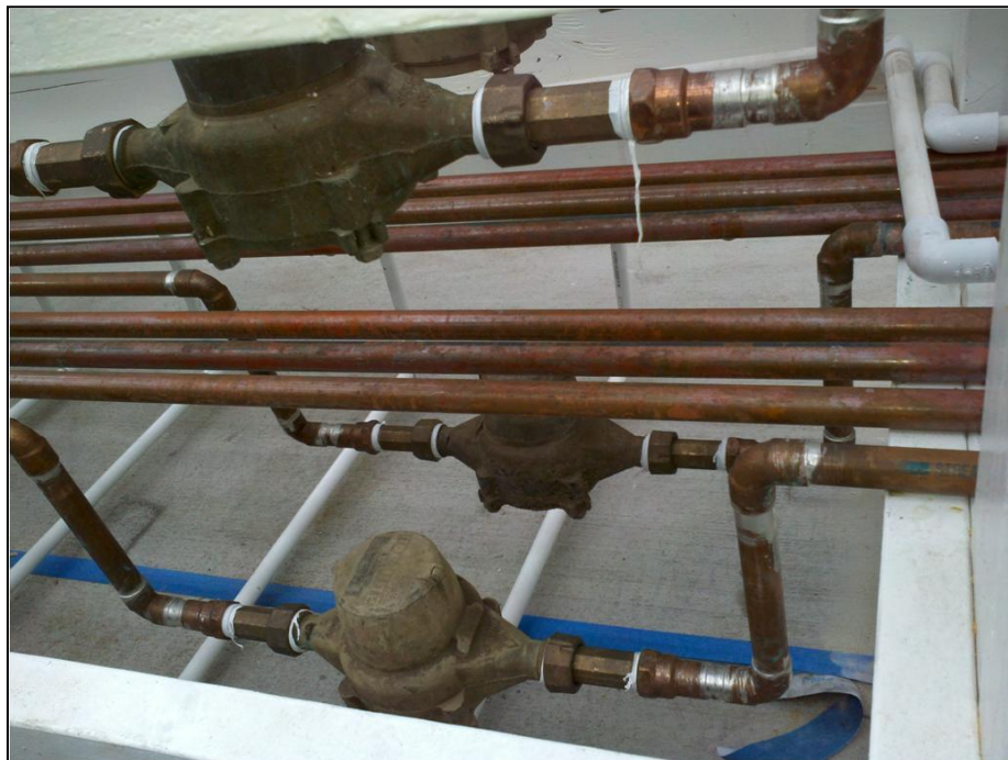
Figure 3-5. CU Pipe Loops (top) and Brass Meters (bottom)
