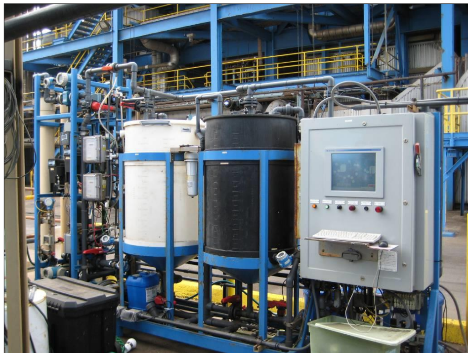
Figure 4-12 Pall Microfiltration System
