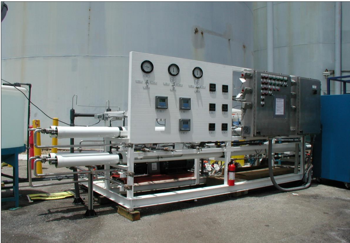
Figure 4-9 Seawater Reverse Osmosis Pilot System
