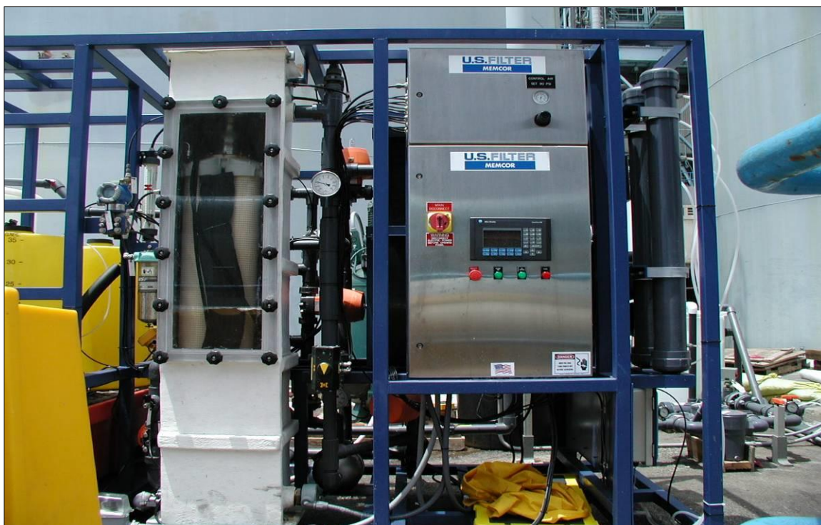
Figure 4-8 Siemens CMF-S Microfiltration Pilot System
