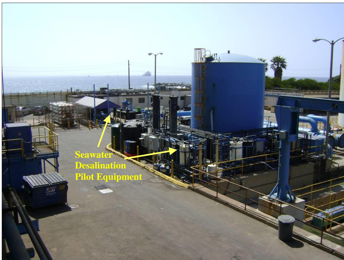
Figure 4-4 Photo of Seawater Desalination Pilot Equipment
