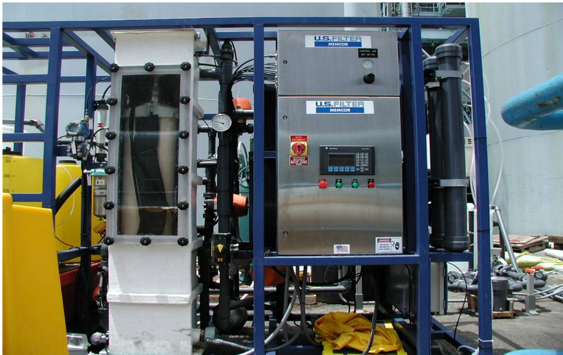
Figure 5 - Siemens CMF-S Microfiltration Pilot System
