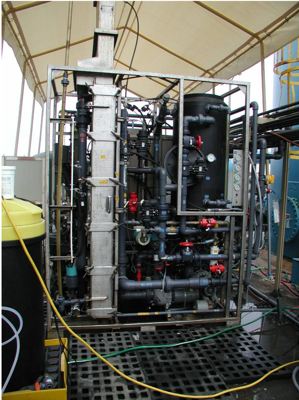
Figure 30 - Zenon ZW1000 Ultrafiltration Pilot System
