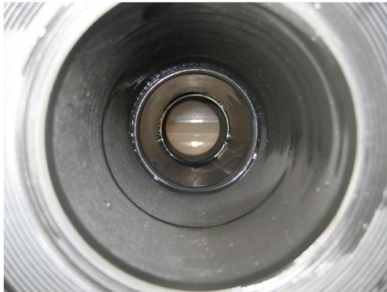
Figure 3-5. Pipe spool B4 (Continuous Chloramine Injection) December 23, 2014. Inlet (top) and Outlet (bottom).
