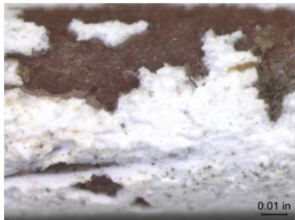
Photo 4-8: Detail view (50x) of coating damage, after cleaning.
