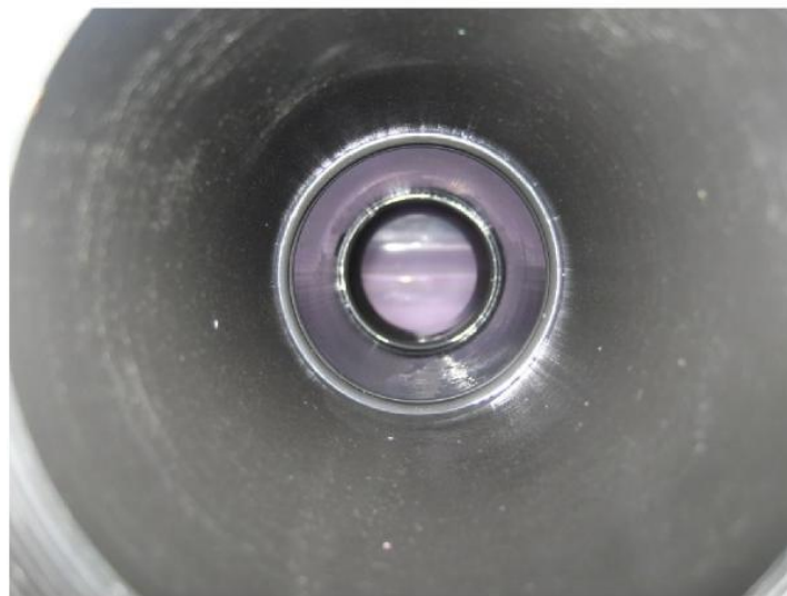
Figure 3-2. Pipe spool B3 (Continuous Chloramine Injection) October 28, 2014. Inlet (top) and Outlet (bottom).
