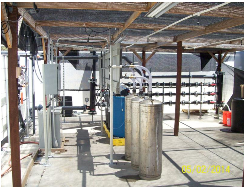
Intake Pipe Testing Facility
