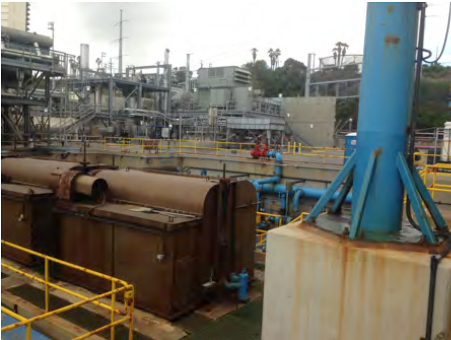
Photo 6: Detail to North of Southernmost Power Plant Components (View Northeast)
