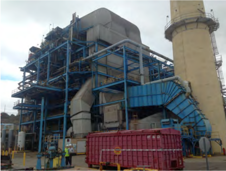
Photo 5: Southernmost Power Plant Components Detail (View Southeast)
