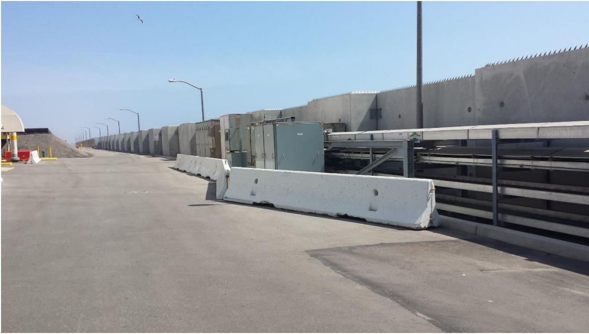
Figure 2: Sea wall at the ESGS North Site, crest elevation =+ 28 ft. to + 29 ft. NAVD
