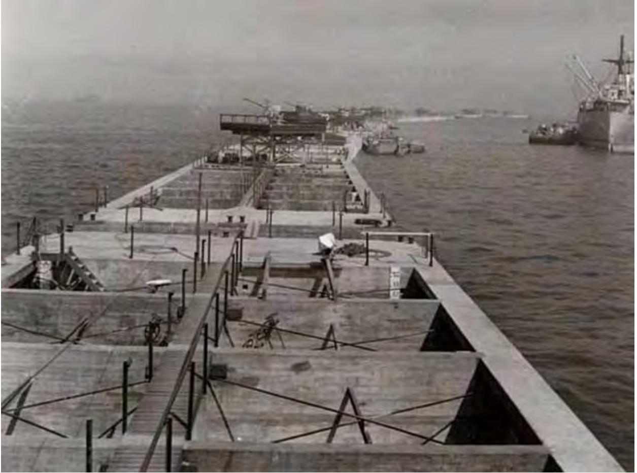
Figure 2.5: Deployment of the Mulberry modules to form a detached breakwater system off Normandy France on D-Day plus 5.
