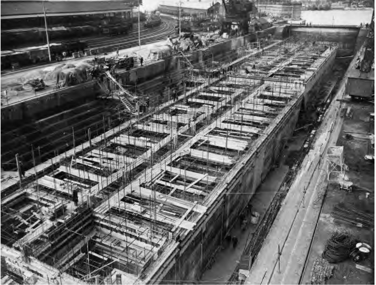
Figure 2.4: Construction of precast concrete boxes used in Mulberry during the Normandy Invasion.
