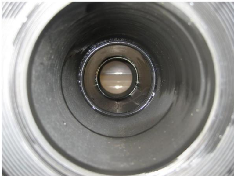
Figure 2. Pipe spool B4 (Continuous Chloramine Injection) December 23, 2014. Inlet (top) and Outlet (bottom).
