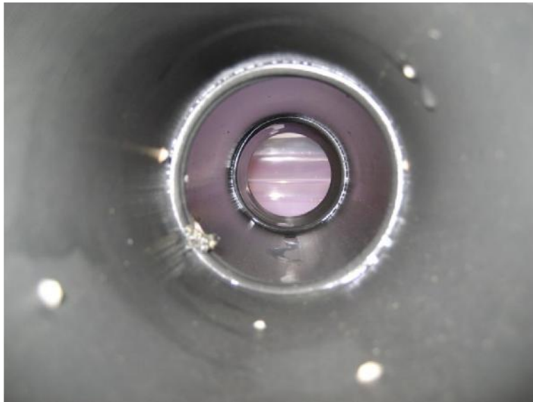
Figure 3. Pipe spool C3 (Shock Chlorination) October 28, 2014. Inlet (top) and Outlet (bottom).
