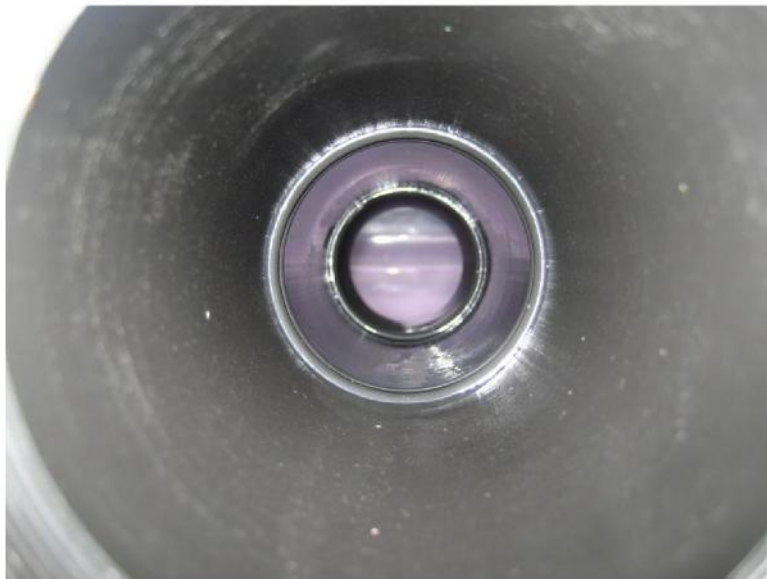
Figure 2. Pipe spool B3 (Continuous Chloramine Injection) October 28, 2014. Inlet (top) and Outlet (bottom).
