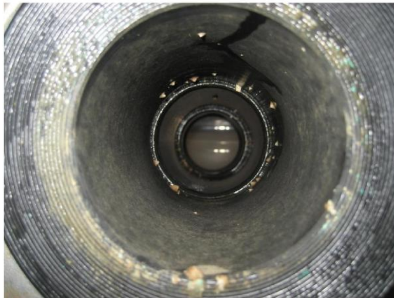
Figure 1. Pipe spool A4 (Control) December 23, 2014. Inlet (top) and Outlet (bottom).
