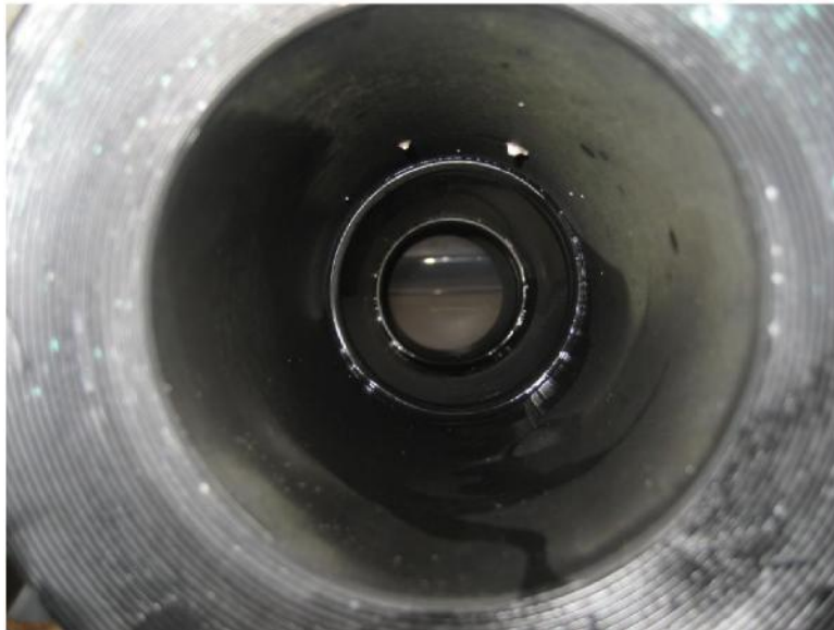
Figure 3. Pipe spool C4 (Shock Chlorination) December 23, 2014. Inlet (top) and Outlet (bottom).
