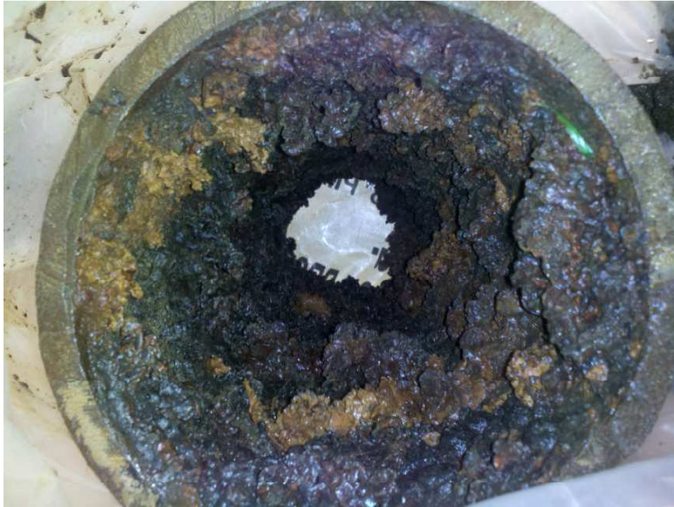
Figure 1: Interior of 6" Unlined Cast Iron Pipe from the Manhattan Beach Distribution System
