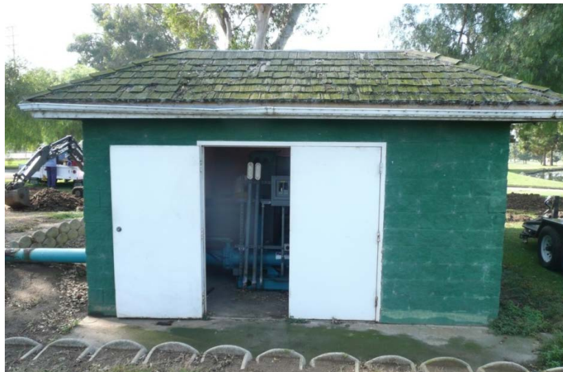
Figure 12. View of Pump House, Chester Washington Golf Course SOURCE: Sapphos Environmental, Inc., 2016
